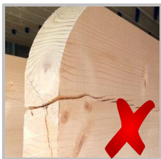
Crack of the board
